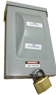
Figure 13. Wind-PV Grid Disconnect Switch in OFF position and locked for maintenance.
