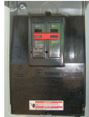
Figure 11. Wind-PV Grid Disconnect Switch in the OFF position, shutting off power to the Inverter.
