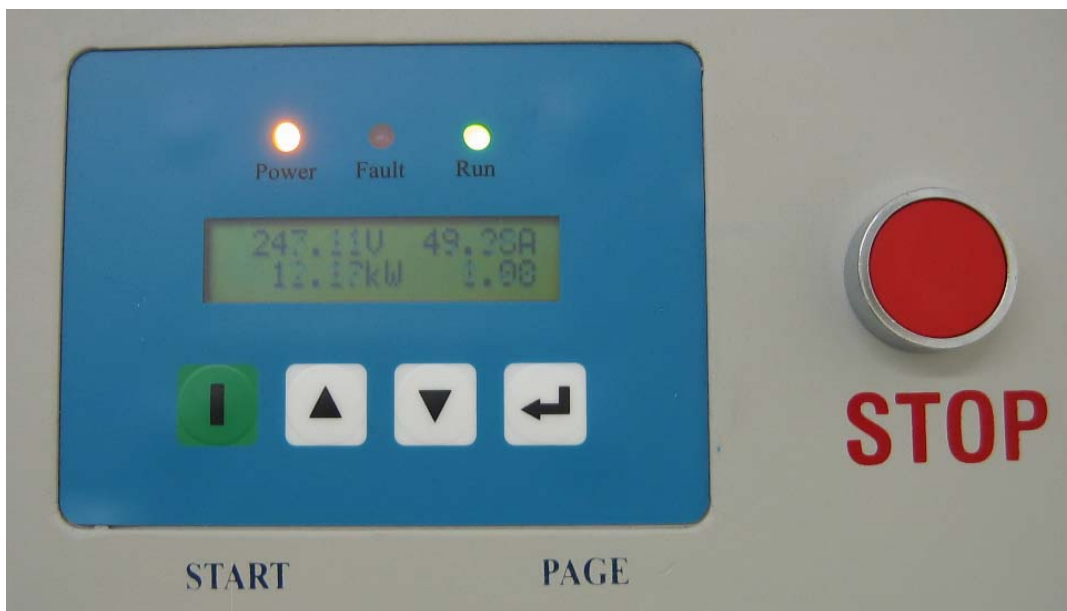
Fig. 4 Inverter Display/Control Panel and Emergency Stop Button
